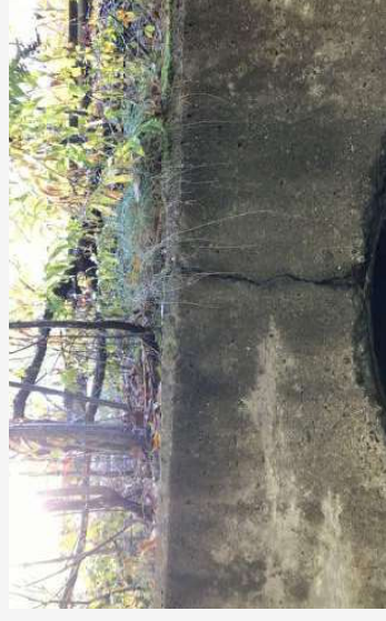
West Headwall – Vertical crack
